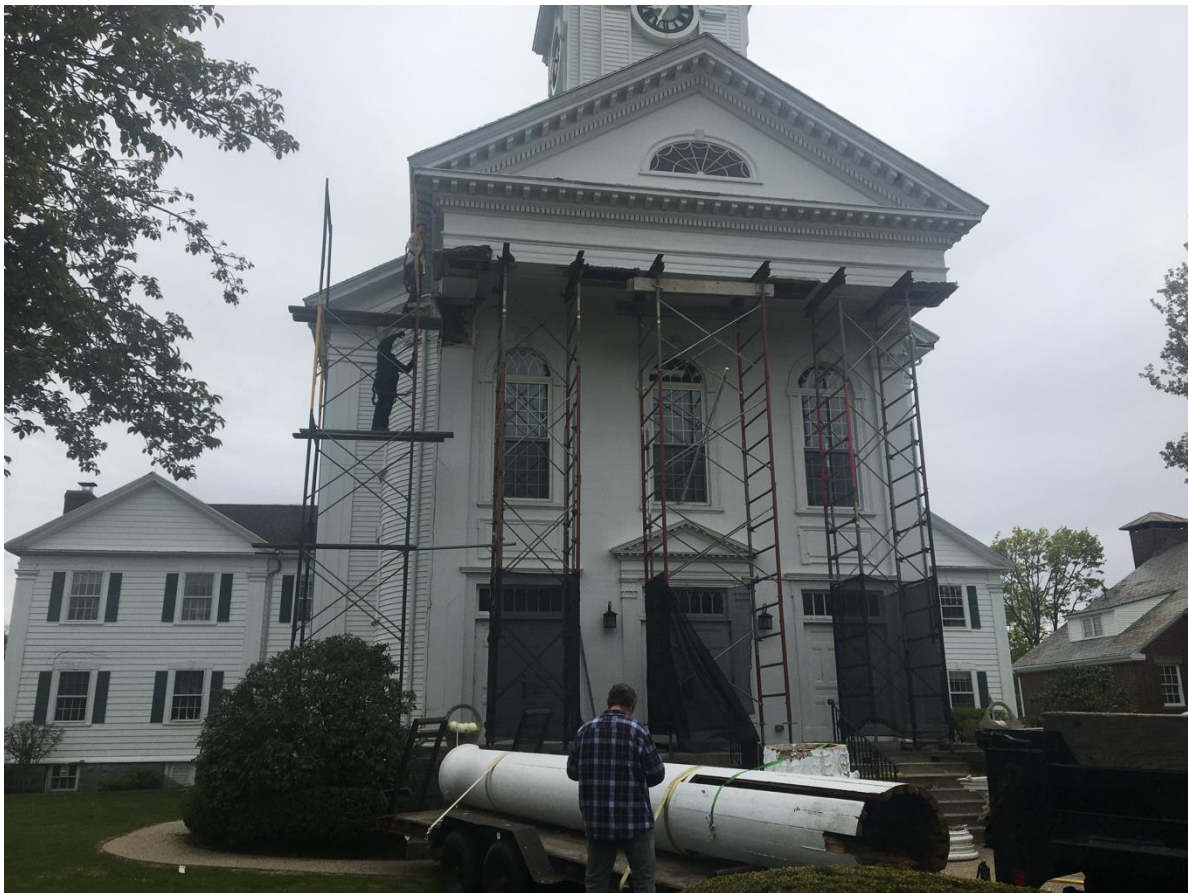
Courtesy of Clif Holbrook: Last of the columns at First Baptist Church in Needham taken down on May 2, 2022
